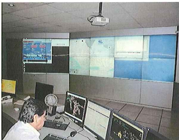
Remote control room at SEDAPAL's main office
