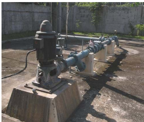
Deep well water source facility
