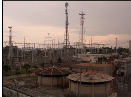
Old substation (Long Binh) still in good condition
