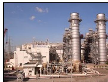
Phu My 4 power plant
