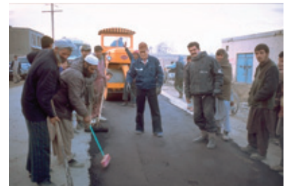
A study team member proceeding with road improvement in an emergency development study (Afghanistan)
