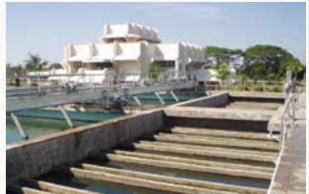
Water supply project in Batangas City in the Philippines: Water Treatment Plant, precipitation system
