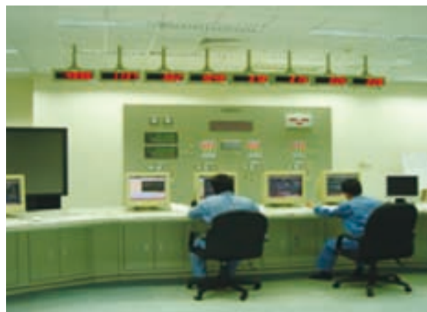
The control room of the Phu My thermal power plant
