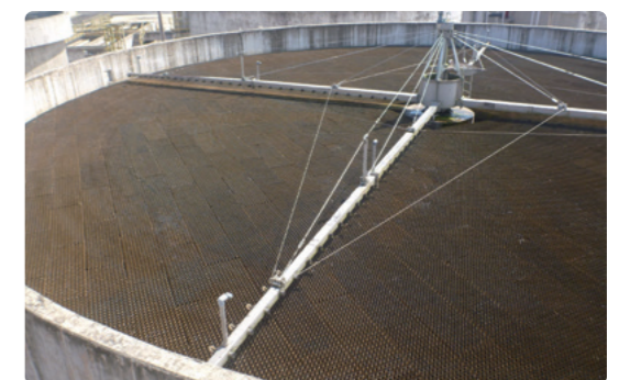
Wastewater treatment plant (trickling filter)
