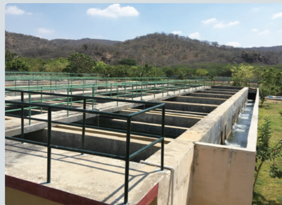
Hogenakkal Water Treatment Plant
