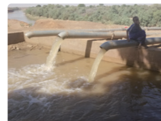
Irrigation facility constructed in Somali Region
