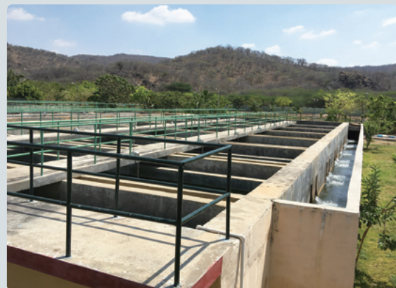
Hogenakkal Water Treatment Plant
