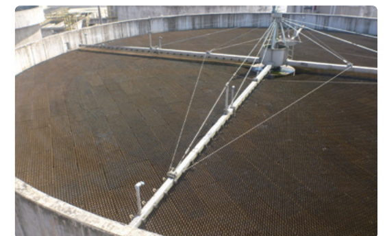
Wastewater treatment plant (trickling filter)
