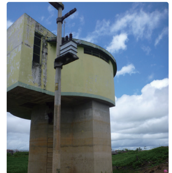
Pumping station constructed by the Project
