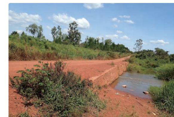
An access road and river crossings and road-drainage culverts improved by the project (Omoro District)
