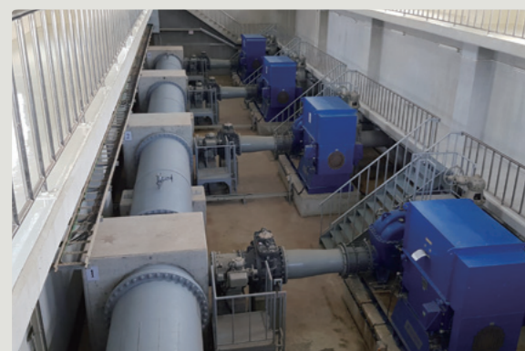
Transmission and distribution pumps installed by the project at the Nyaungnabin First Phase Water Treatment Plant
