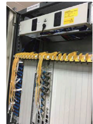
Supply-side broadband access facilities
