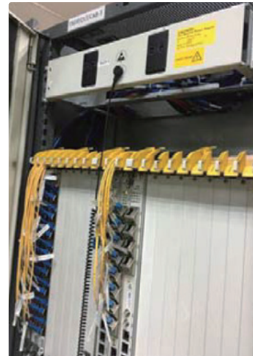
Supply-side broadband access facilities
