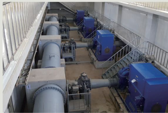
Transmission and distribution pumps installed by the project at the Nyaungnabin First Phase Water Treatment Plant
