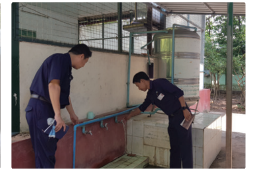
The project improved water pressure and quantity at a primary school in Yankin Township
