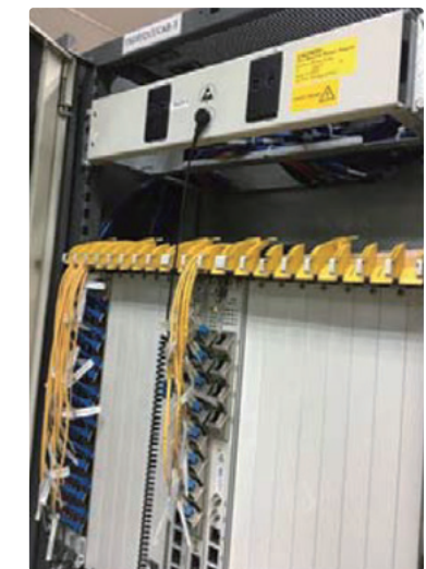
Supply-side broadband access facilities
