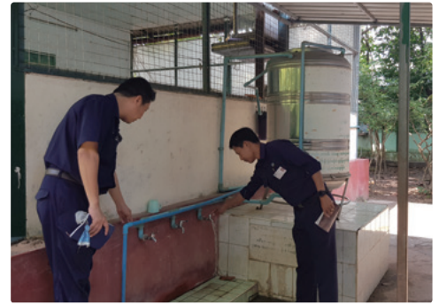
The project improved water pressure and quantity at a primary school in Yankin Township
