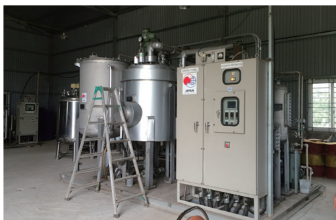
Analytical equipment provided by the SATREPS project at VNU
