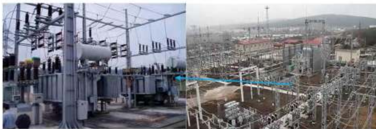
Plate 3.15: A Typical AIS Substation (with transformers zoomed in)
