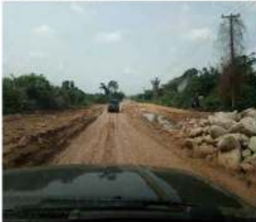
Plate 4.55: Devastating state of the major road (Papalanto-Shagamu) to these communities
