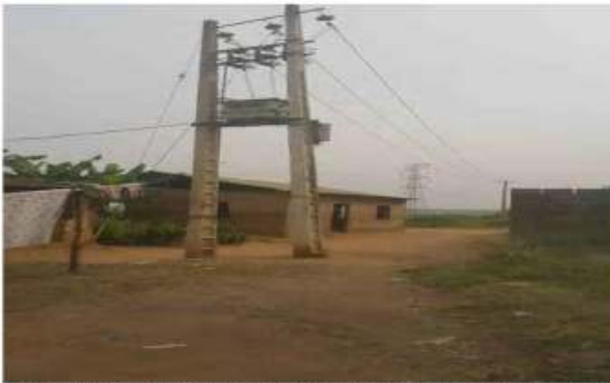
Plate 4.53: Electricity line and Transformer at Soderu Community
