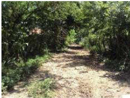
Photograph No. VI.27. Ballast Road in poor conditions near station 9+170
