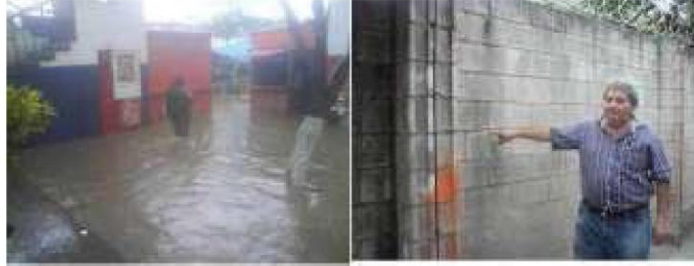
Photograph No. X.3. Images of tropical storm Agatha, in the area of the school in Colonia Carrillo, where flooded areas are shown. The school principal shows the level the water reached
