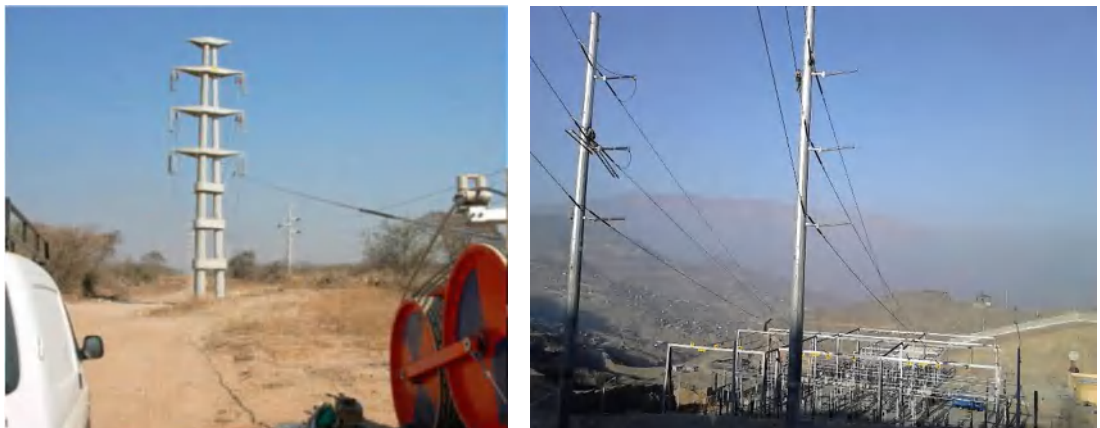
Figure 50 – Cable tensioning equipment and line next substation
