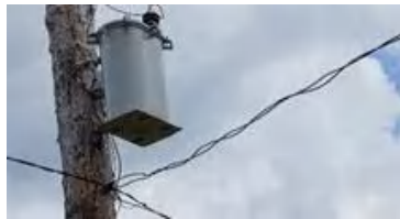
Photo: electrical installation.
