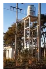
Water System, Jhuguá Po’i
