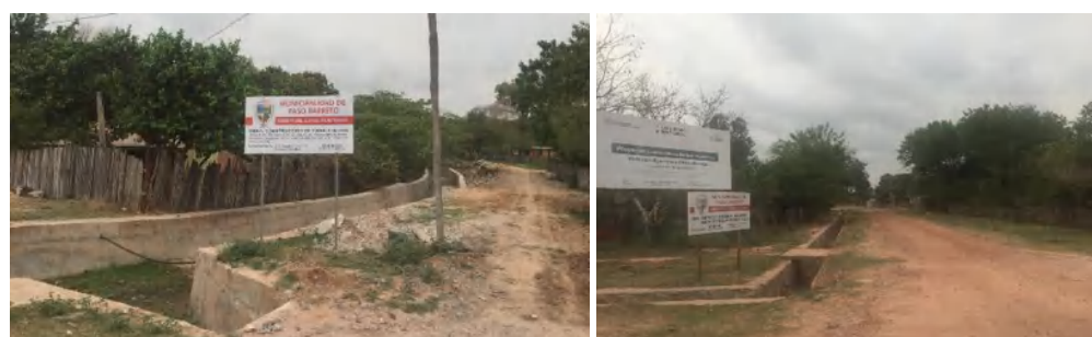
Figure 35 – Construction of the Canalization System and the Storm Drain Channel - Paso Barreto
