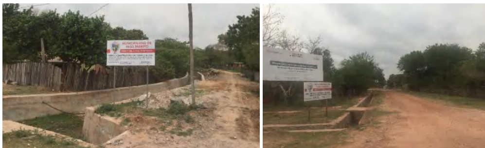
Illustration 1. Construction of the canalization system and the storm drain channel - Paso Barreto
