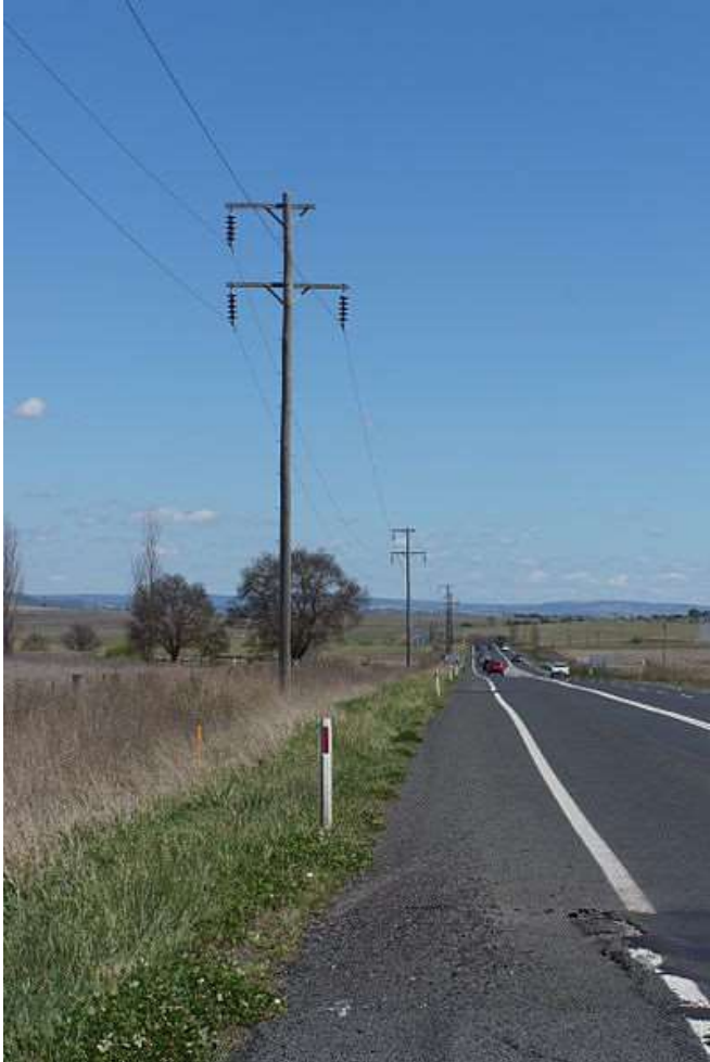
66 kv Transmission line
