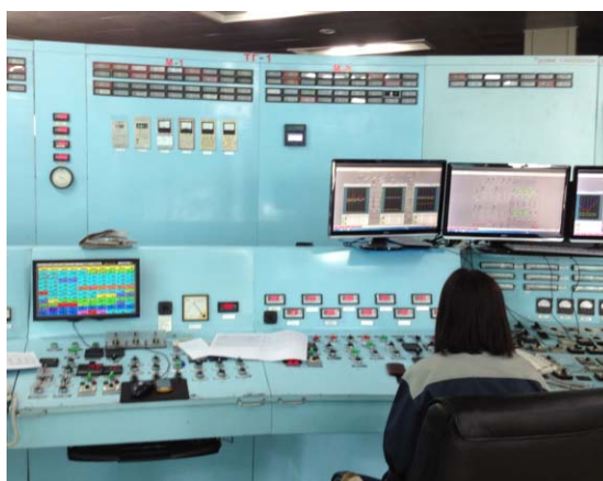
Fig.4.2-20 Turbine Control Panel in CCR
