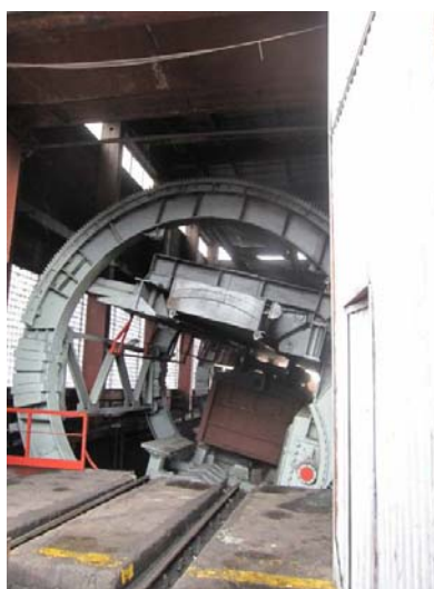
Fig.4.2-29 Coal Unloading Facility of TPP4
