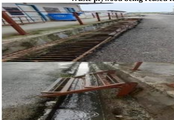
Waste steel rebar used for making mesh for covering the drain and waste steel material used for making stairs in labour camp, etc.
