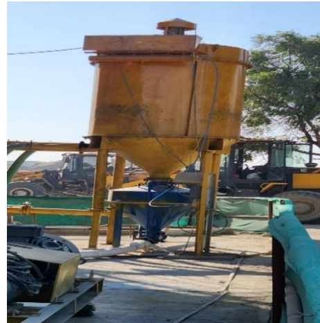
Dense Phase System in C6 package
