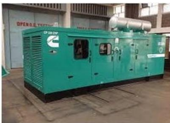
Acoustic Enclosure on DG Sets
