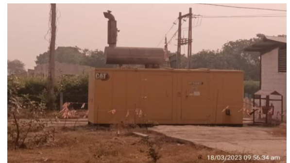
CPCB compliant DGs are used having sufficient stack height and placed at upwind direction in the PCY 264
