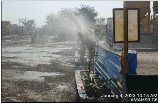
Use of RO rejected water, permanent mechanism made for water sprinkling at batching plant area at Ch 434, C6 Package
