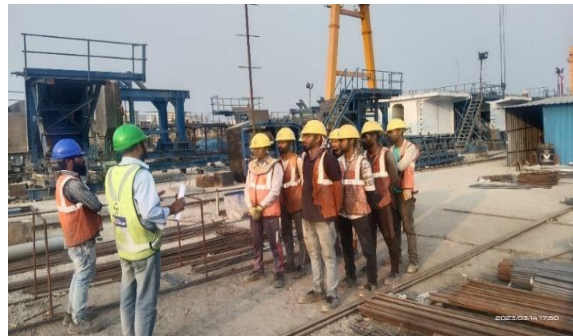
Training Provided to the workforce about Noise and Air Pollution at Ch. 217
