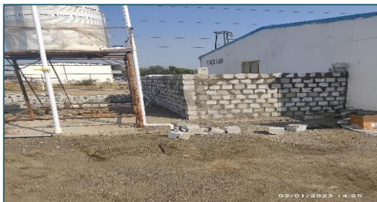
Tested QC cubes are used for making garden wall, bund wall, drain etc. in all section and tested concrete cube is used for making tree guard in all section in C6 Package.
