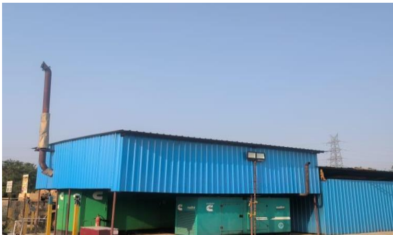
DG with adequate stack height at Ch. 168
