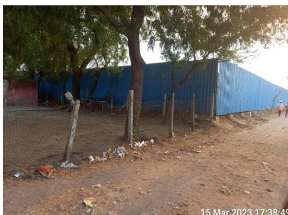
Metal sheets are provided along the project boundary near the sensitive & residential area at Ch. 260
