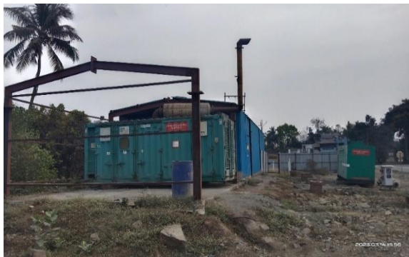
Adequate Stack height on DG set at Ch. 217
