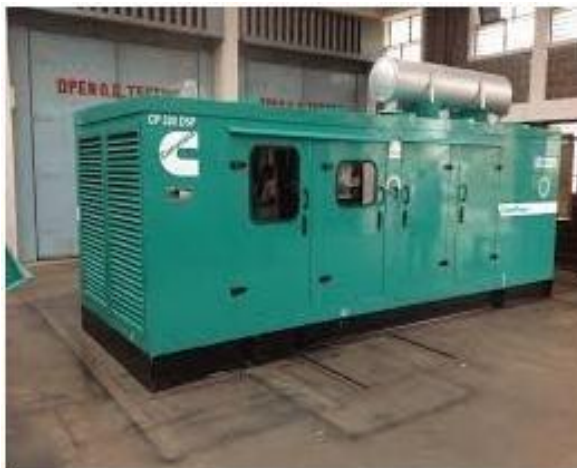
Acoustic Enclosure on DG Sets
