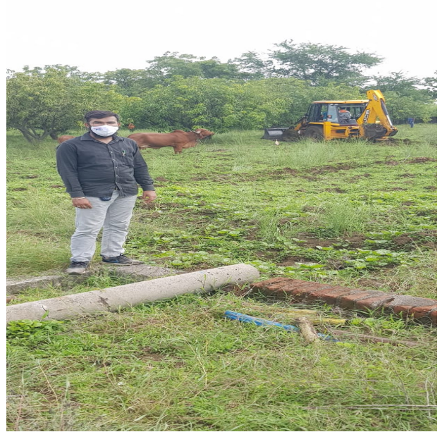
28 th June 2021 Alignment clearance at Pasodara and Tarsadi village of Surat District
