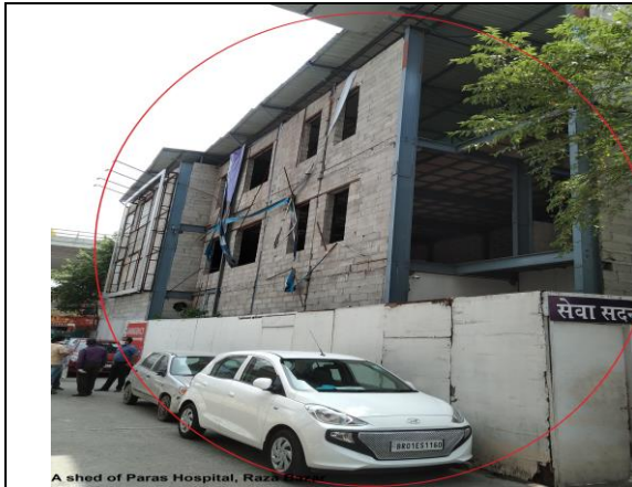
RB6 – Affected structure of Raja Bazar
