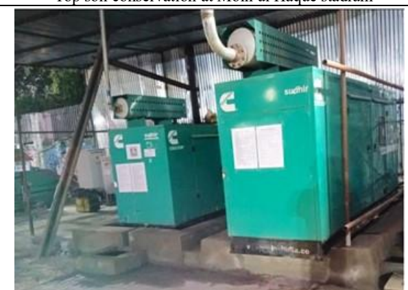
Use of silent Diesel Generator set with appropriate stack height
