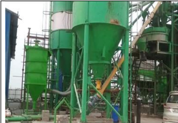
Dust collector in batching plant
