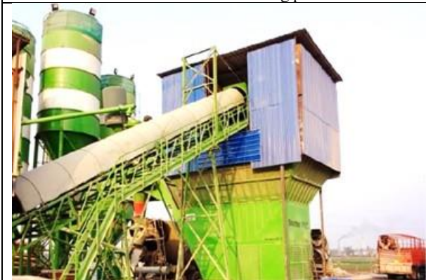
Covering of conveyor belt
