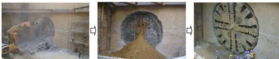
Case4 (Retrieval: The diaphragm wall was demolished by breaker up to soil face reinforcement. Soil improvement of the diaphragm wall was not required.)
