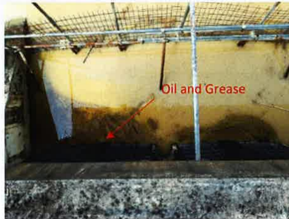
Figure 1 Found the oil and grease in SW-1 (retention pond discharge)
