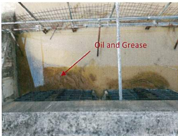
Figure 1 Found the oil and grease in SW-1 (retention pond discharge)
