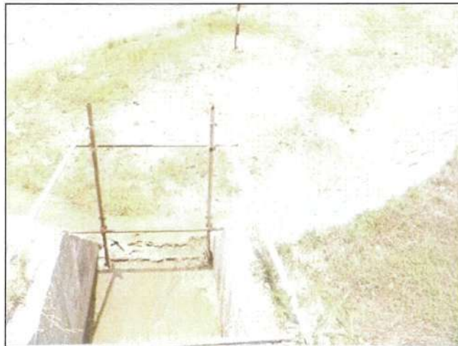
There is no water at SW-5
