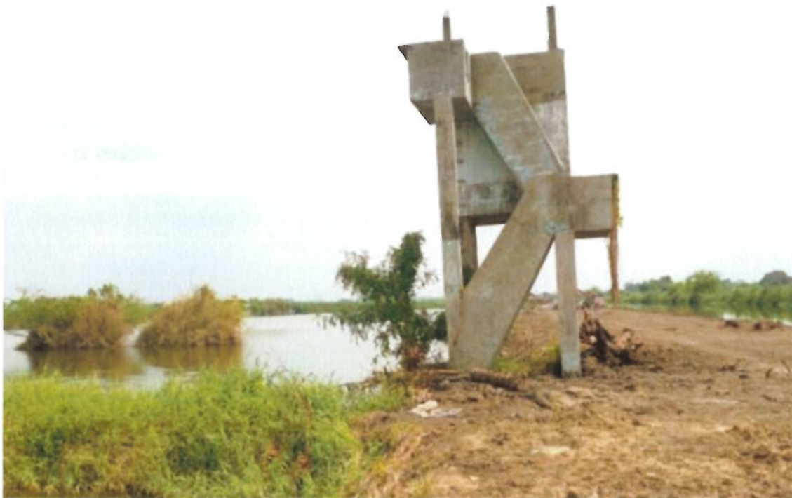
Location: Brgy. San Matias, Sto. Tomas, Pampanga Date: July 6, 2021 Description/Comment: Affected Structure owned by Mr. John Florendo located inside the PNR ROW
