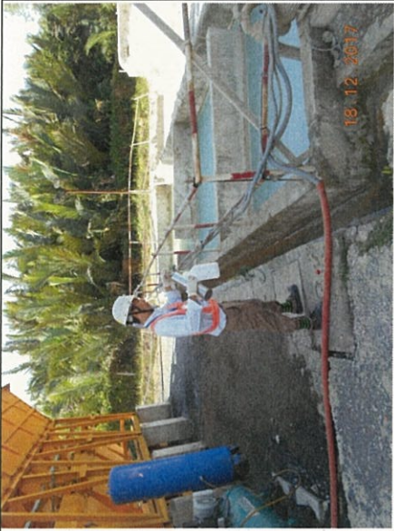
Sampling waste water at WW1
