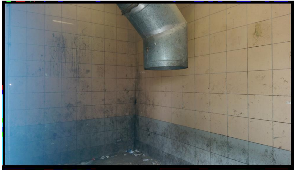
Photo No.14 shows the assembly room of solid wastes
