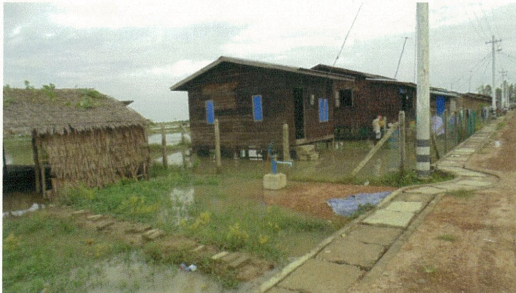
Photo 4 – Flooding around a water pump.
