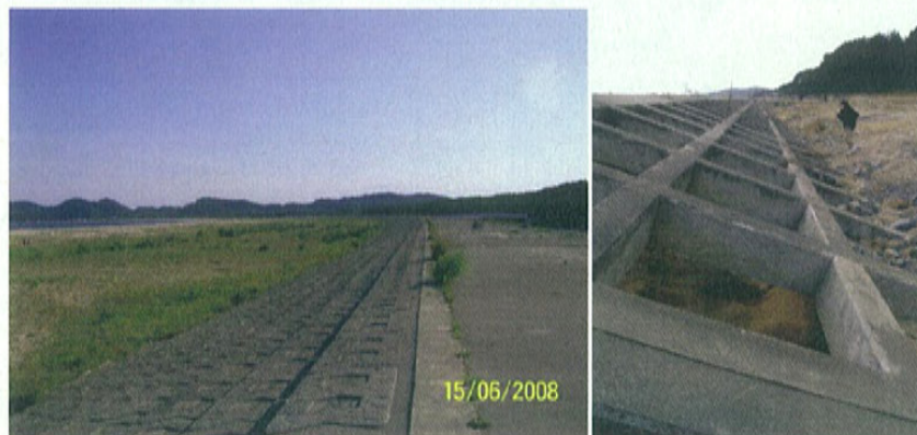
Fig. 6 Seawall along Nobiru coast before and after tsunami
