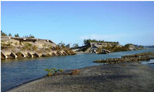
Destroyed Sea Dike, Isobe, Soma City (Mar. 29, 2011 by Matsumaru)
