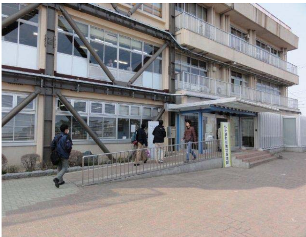
Reinforcement of the building was done in recent years Photo 4 Shichigahama City Government Building
