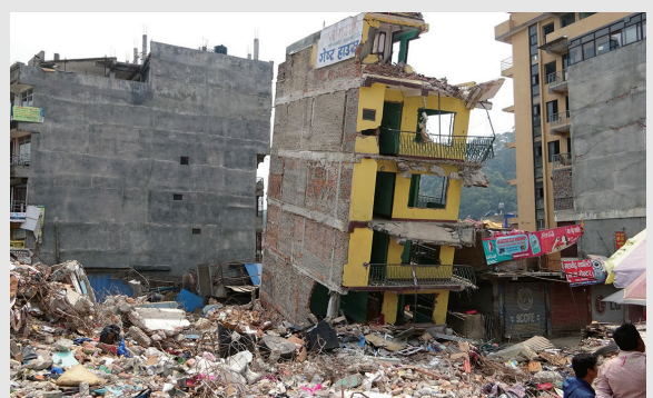
Damage of the 2015 Nepal Earthquake Disaster
