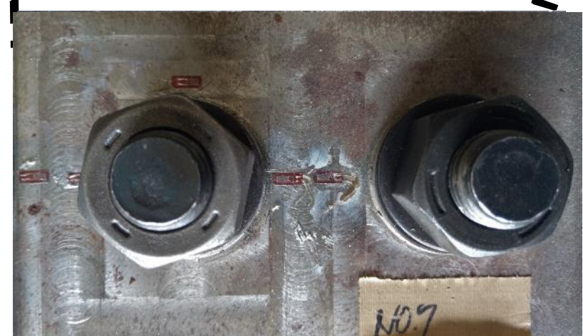
Uniform corrosion case: U
