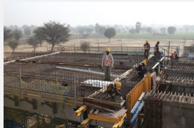
Work in progress at the Jaipur site of Dedicated Freight Corridor Project
