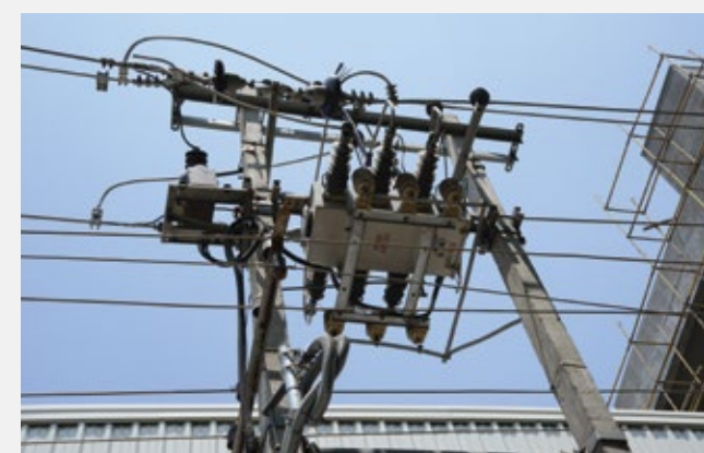
LBS automatically isolate faulted sections of electrical distribution system, Bangalore Distribution Upgradation Project
