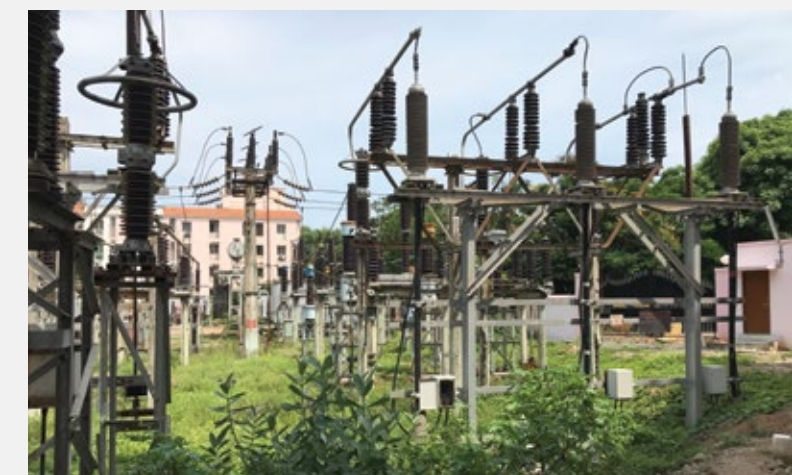
Sub-Station to improve electricity supply, Tamil Nadu Investment Promotion Program
