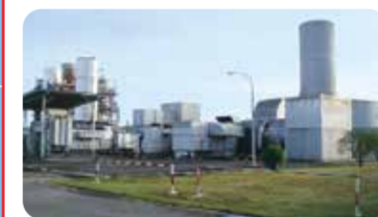
Construction of gas turbine power generator with 33.2MW capacity in Patau-Patau power station. (Completed 1995)
