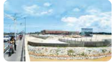
Development of basic infrastructure such as rural roads, water supply facilities, land development etc. (Completed 1992)
