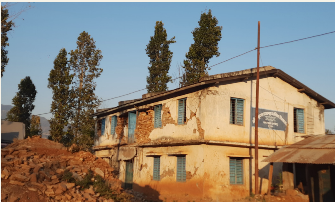
Damaged structure of Shree Tribhuvan Secondary School ,Bheri Municipality, Jajarkot (2024)
