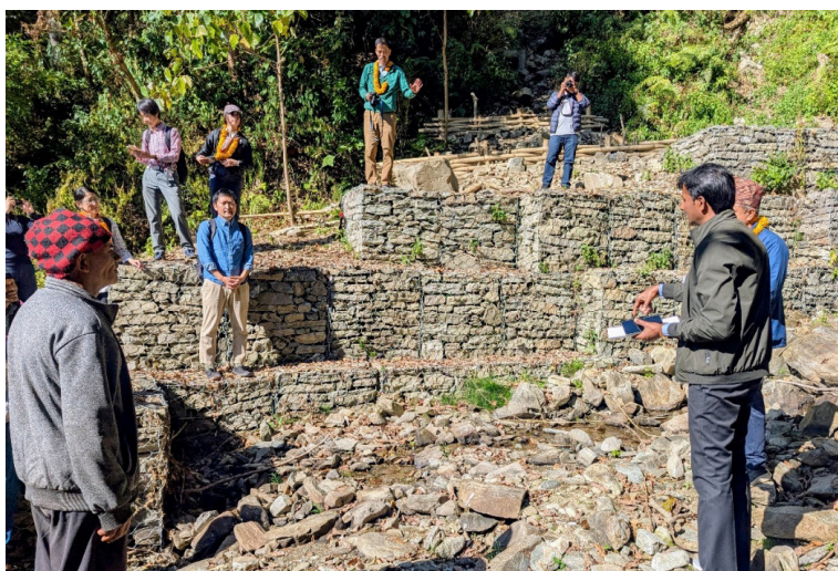
SWMO Chief, Parbat, explains how learnings from the project trainings are being utilized in constructing local gabion check dams and bioengineering techniques
