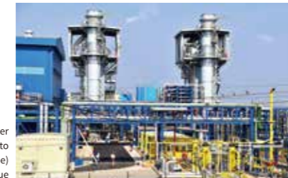
Gas Fired Combined Cycle Power Plant Development in Maputo (Mozambique) Photo : Electricity of Mozambique
