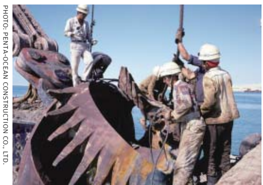
Workers replacing a 3 m diameter cutter blade, which attaches to the end of the ship's rudder.
