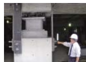
A seismic-isolation device attached to a pillar at the Arakawa City Office.
