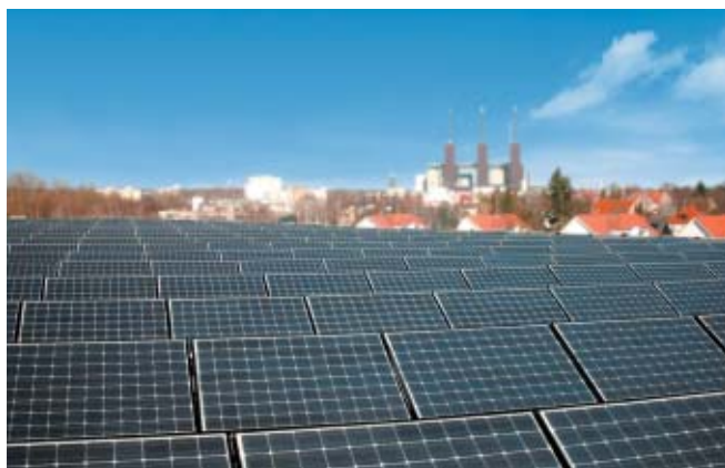
HIT solar cell modules installed in the Berlin City Gymnasium, Germany (System capacity: 40kW; Design/Construction: Schoenau AG)
