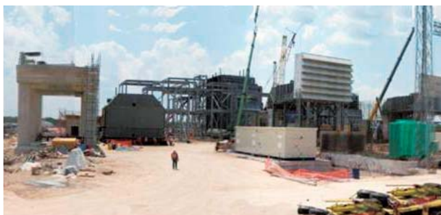
Construction work in the Valladolid Power Project where Japanese firms have participated
