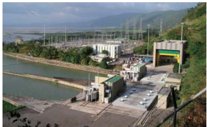
A facility in the CBK Power Project whose concession were acquired by Japanese firms
