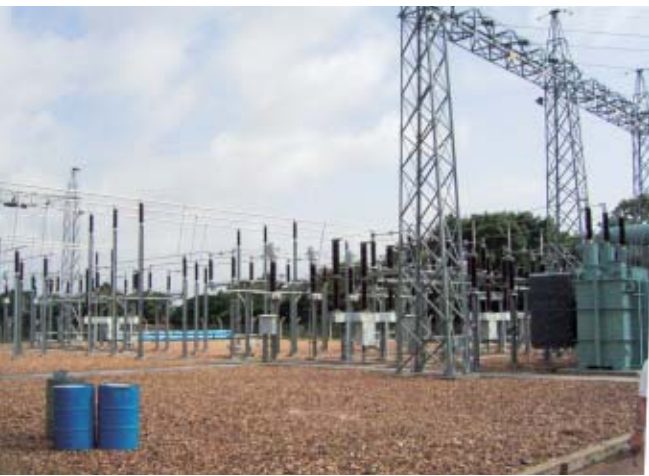
A substation to be expanded by ODA loan (Laos)
