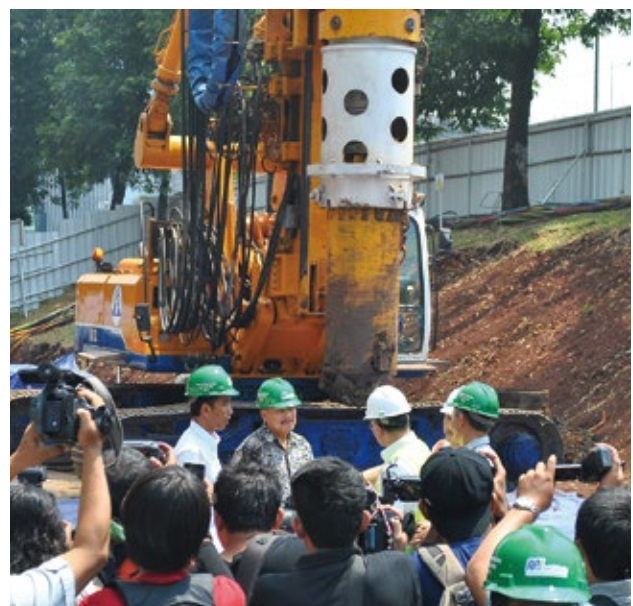
Groundbreaking ceremony for the North-South line (ODA Loan) of the Jakarta Mass Rapid Transit (MRT), which is expected to help relieve the capital's traffic jams.
