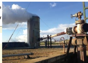
Gas exhalation test in Guanacaste province, Costa Rica. Utilization of Japan’s geothermal technology is expected.
