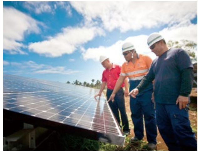
Installation of a micro-grid system under Grant Aid in Tonga
