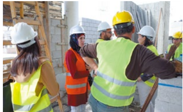
Palestine: A woman engineer teaching how to supervise construction work in the Refugee Camp Improvement Project
