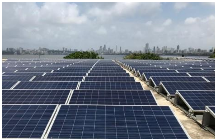
(Picture 1) Solar Power Project financed by TCCL
